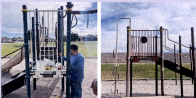
Protective railings were installed at playgrounds due to removal of broken slides.
