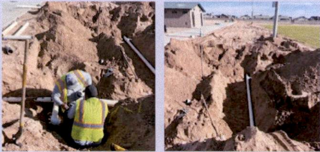
4-inch pipe was relocated, and a 3-inch line was installed at the East Community Park.
