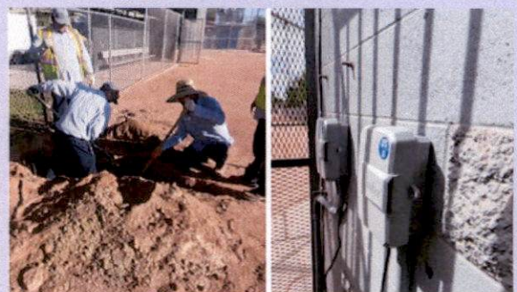
F2 & F3 irrigation timers were relocated.
